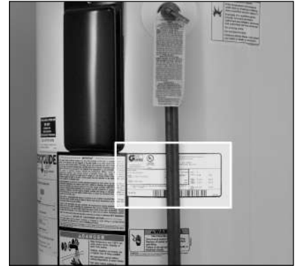
Figure 18 - The water heater’s electrical requirements can be determined from the data plate.
